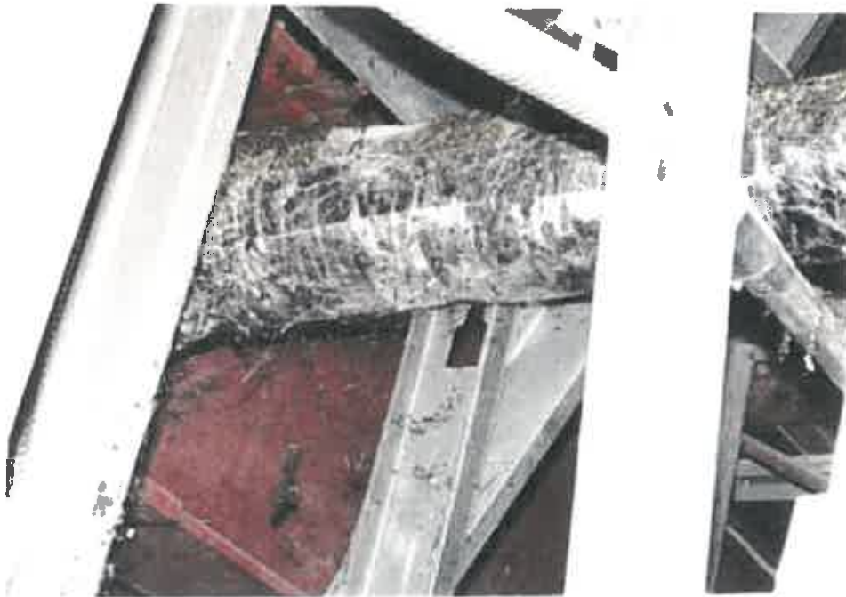
Photo 10: West Club Area, bat guano on ducting near column G40.
