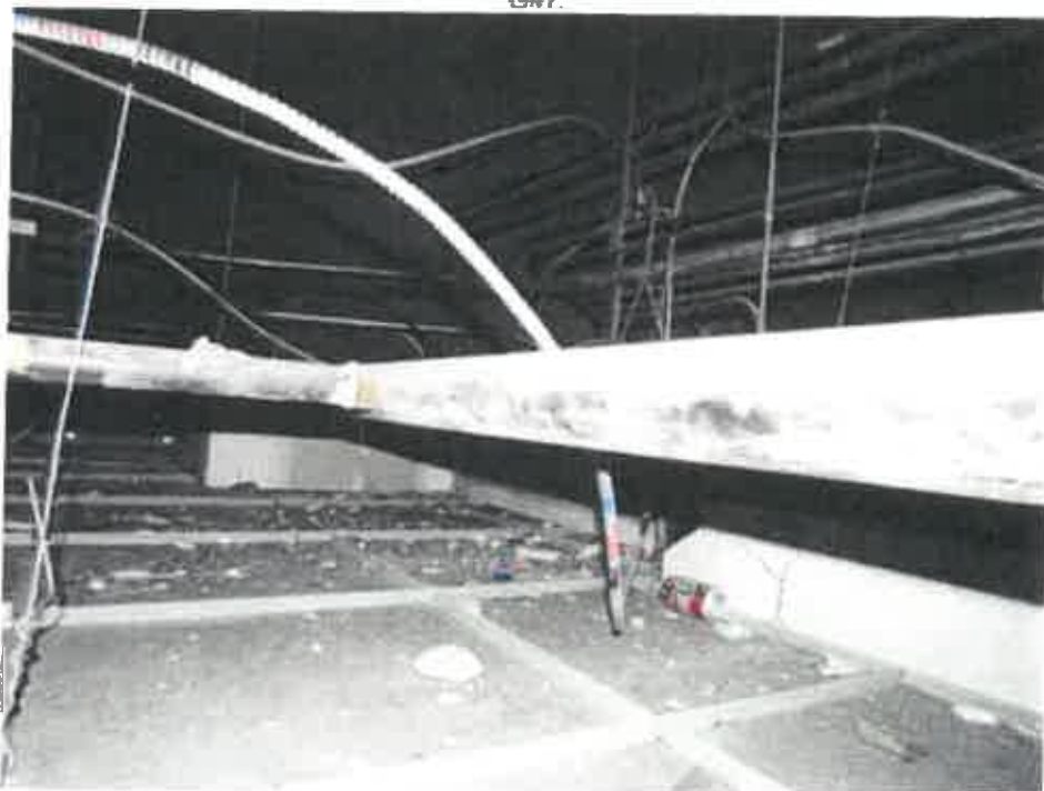
Photo 16: West Club Area, view of debris mixed with some bat guano on ceiling tiles above the concession area near column G49.8.
