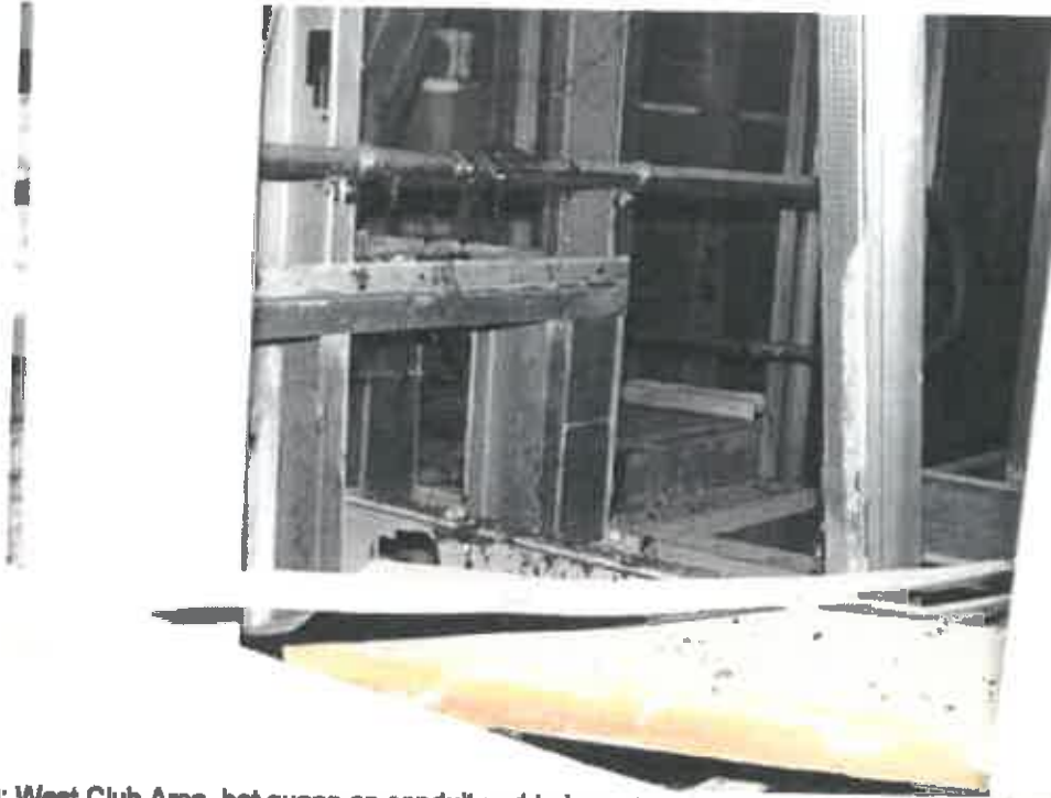
Photo 9: West Club Area, bat guano on conduit and ledges close to expansion joint near column G40.
