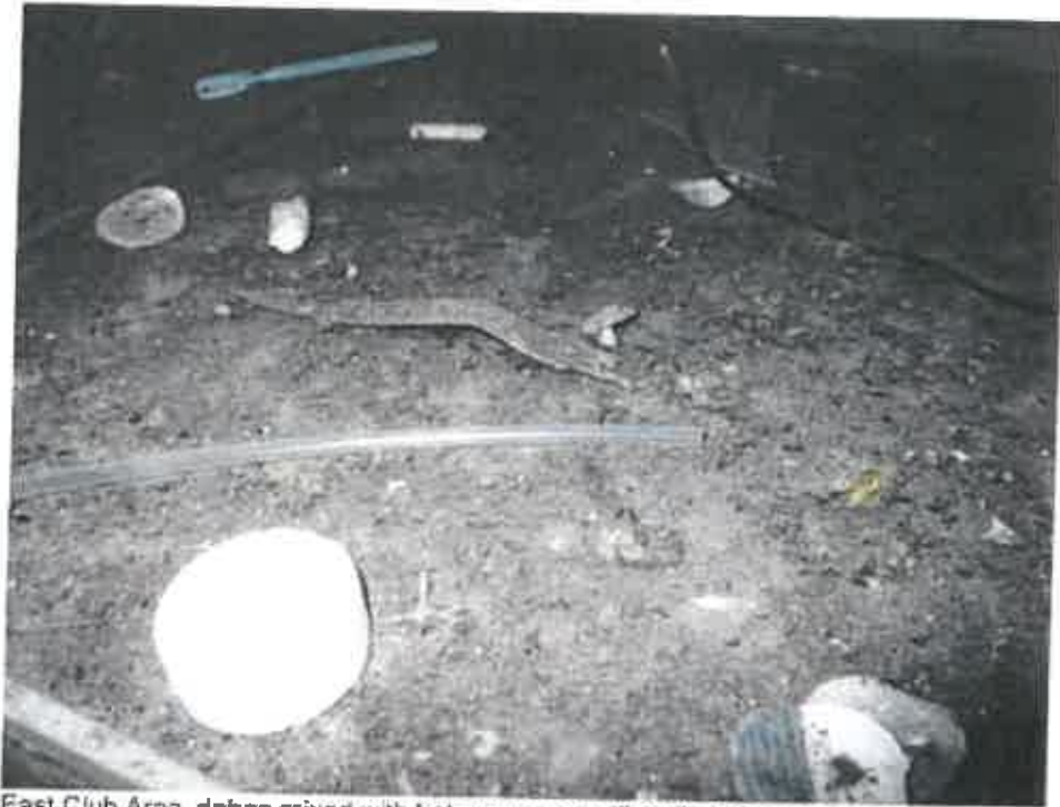
Photo 7: East Club Area, debris mixed with bat guano on ceiling tile in food concession area near column G16 8, associated with vertical smoke evacuation shaft.
