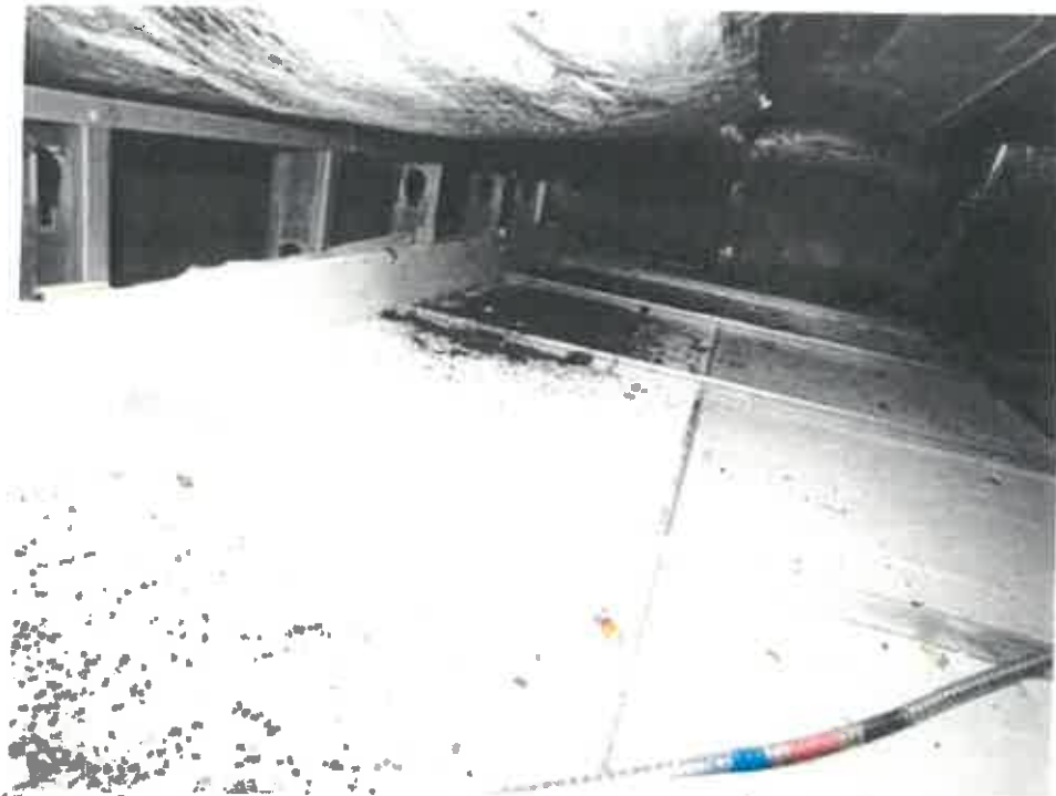
Photo 15: West Club Area, view of bat guano on ceiling tiles looking from column H47 towards column G47.
