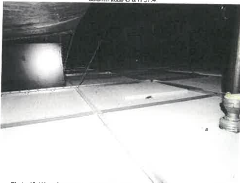
Photo 12: West Club Area, sparse bat guano on ceiling tiles near column G43.
